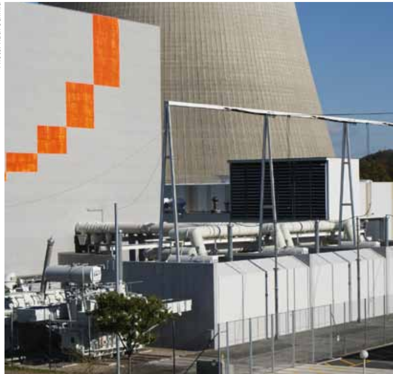
Three transformers form the unit transformer; the fourth one on the left is kept as a standby transformer.
