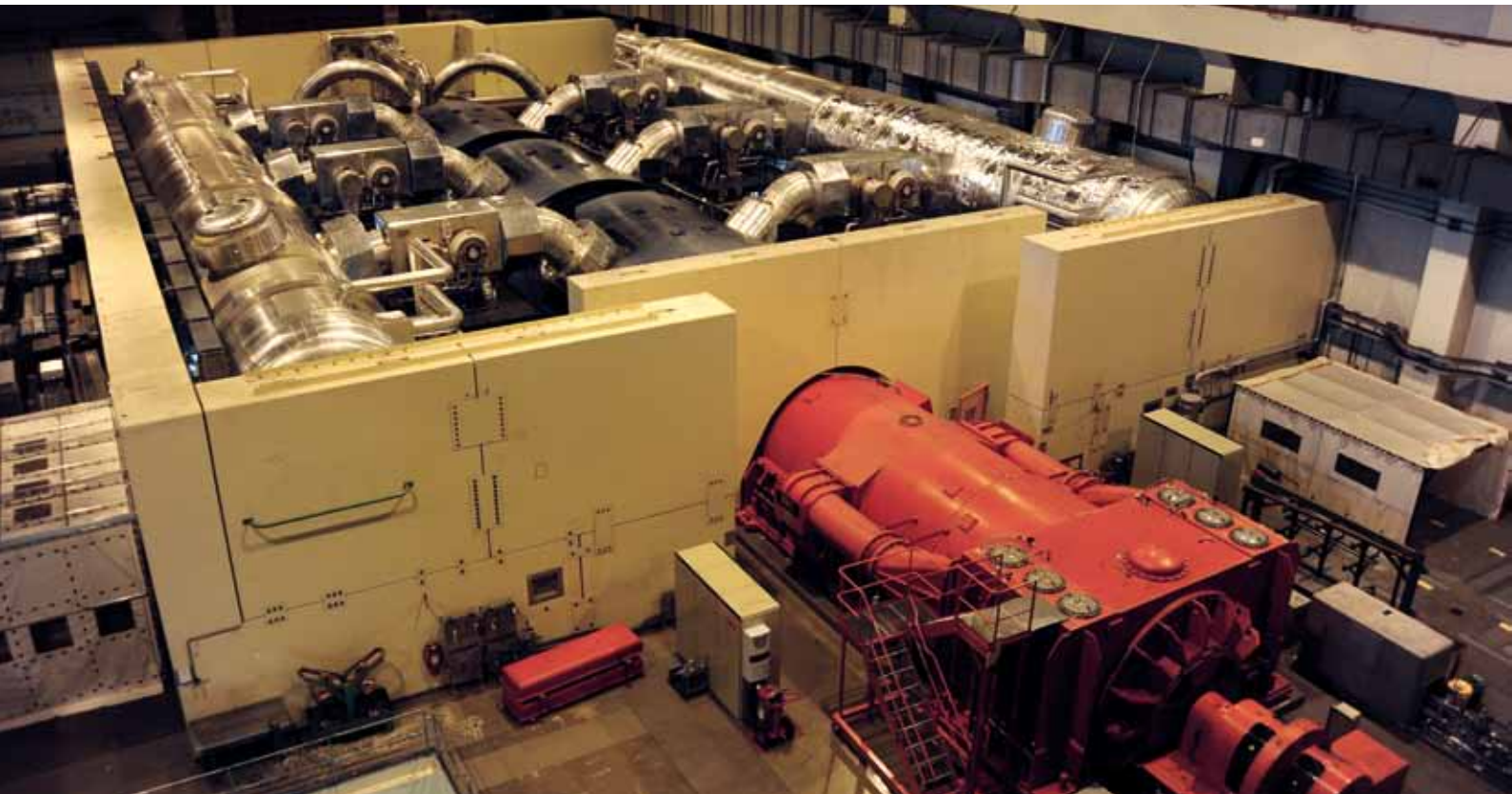
The high-pressure and low-pressure turbines are mounted along the same axis as the generator; the water separator / reheater can be seen to the left and right.
