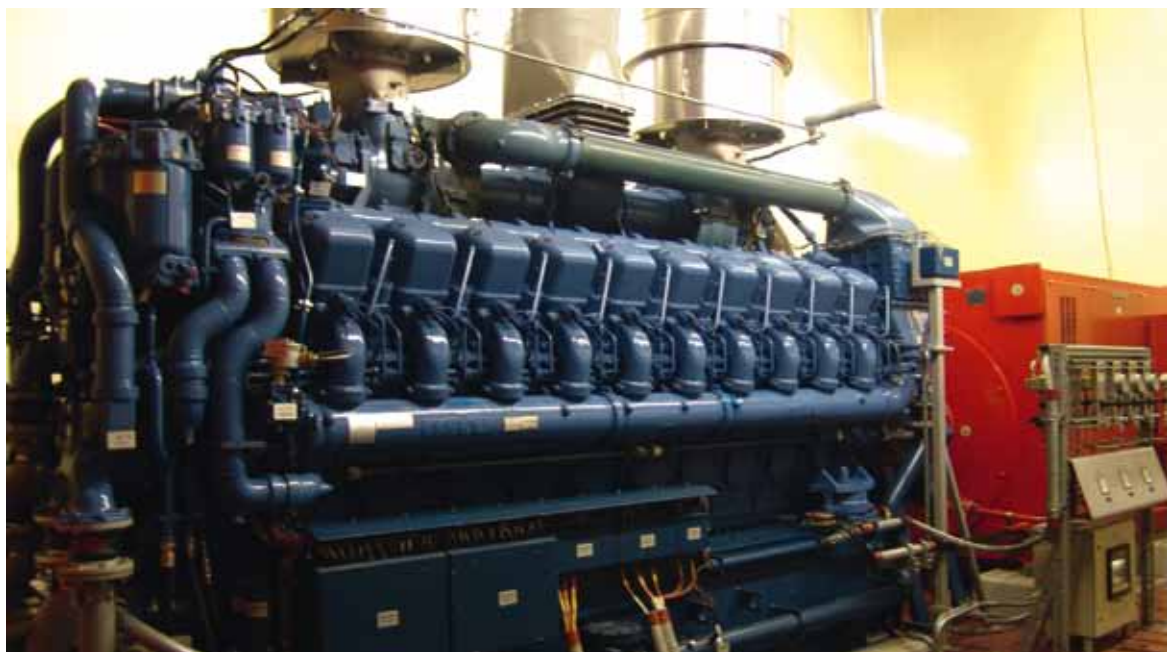
The 20-cylinder engine of an Emergency Diesel Generator.
